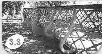
YARRAPARK FOOTBRIDGE Repairs: Jolimont Built: 1970 $40,000 to replace damaged planks and asphalt
