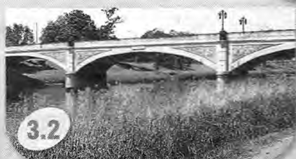
MORELL BRIDGE Repairs: Sth Yarra Built: 1899 $473,000 to patch up and paint
